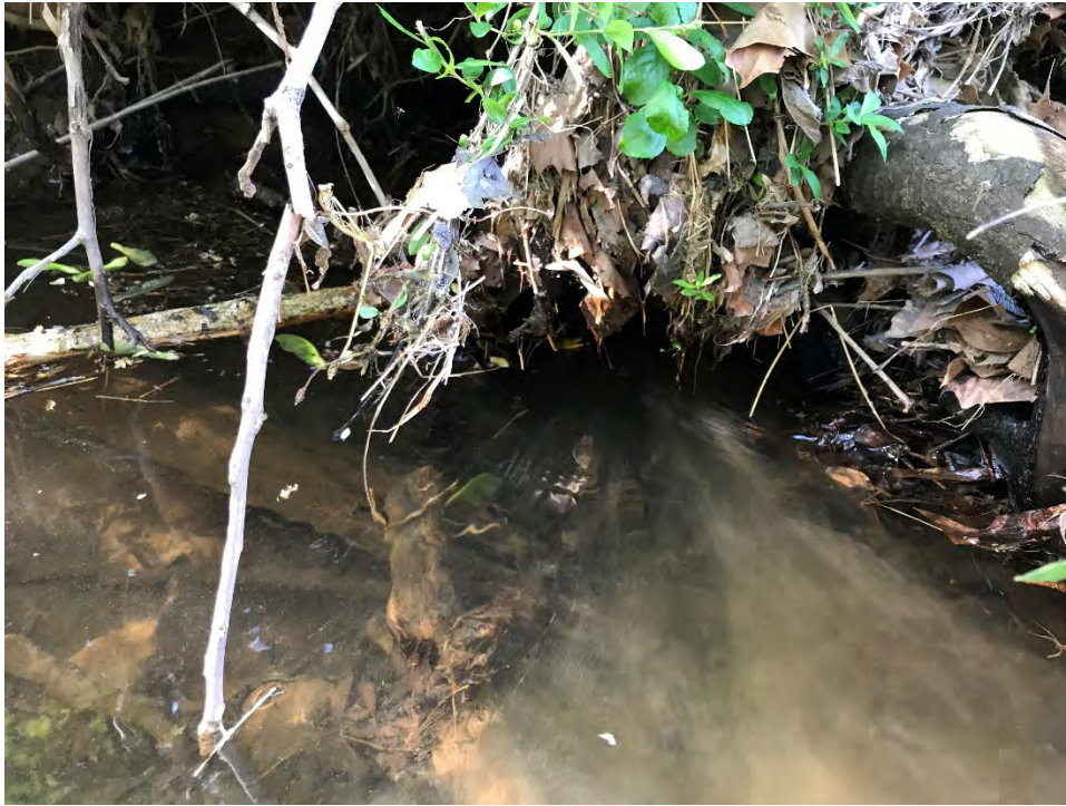
Figure 39: Drain pipe inflow located in active channel (facing right bank)
