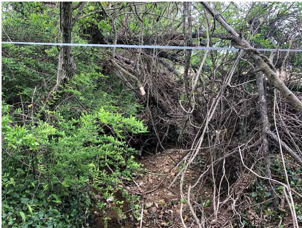
Figure 45: Upstream end of longitudinal profile 8 in Intersection Tributary with debris jam
