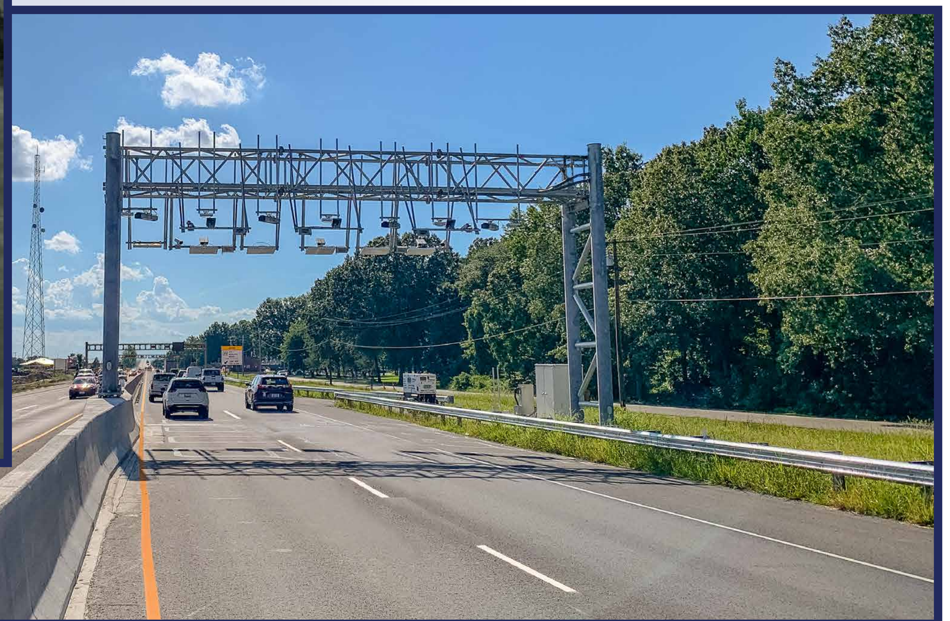
New overhead gantry for all-electronic tolling, 2022
